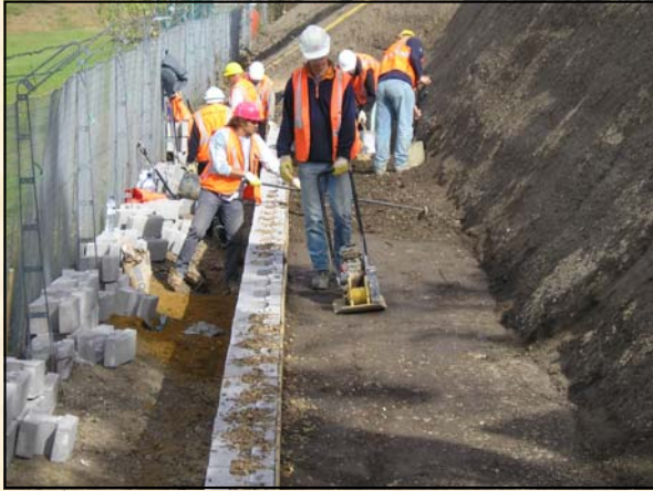
Compaction immediately behind the structure is carried out with vibrating plates only, to limit movement of the block fascia
